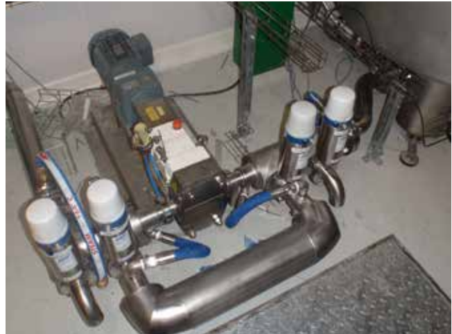
Pumped liquid - glucose Syrup 80 °Bx Pump - LPX50-1 with heated cover and double mechanical seal
